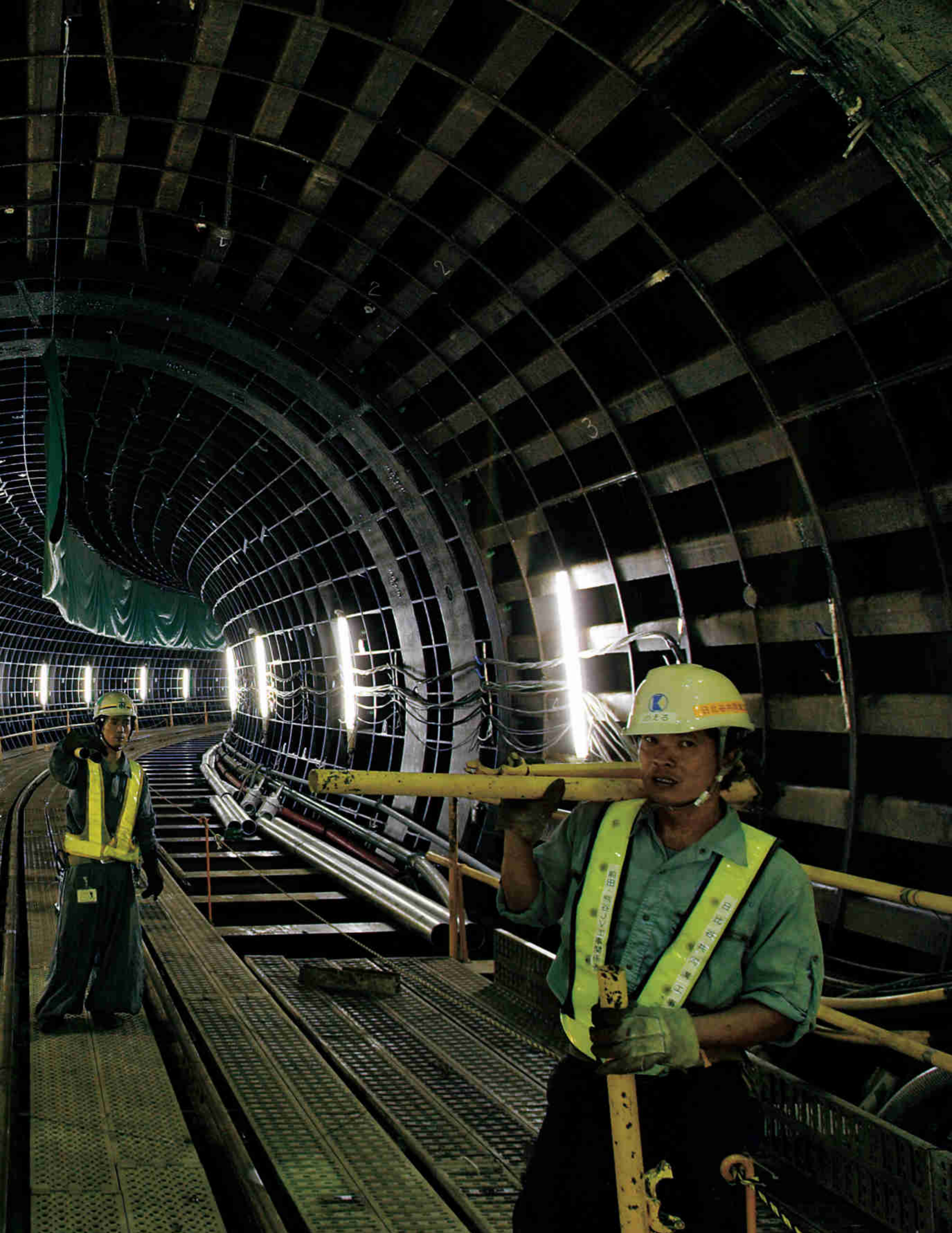
Deep under Tokyo's streets a construction crew prepares a quake-resistant duct for the city's water, electricity, telephone, and sewage lines. By minimizing damage to the main utility lines, the tunnel should allow services to be restored quickly after an earthquake.
